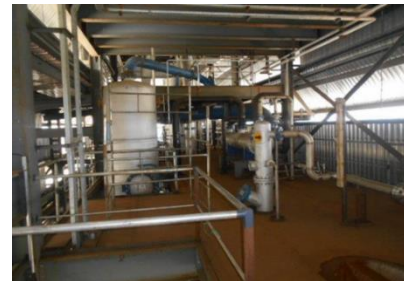
Figure 7 – Oil Extraction Facility
