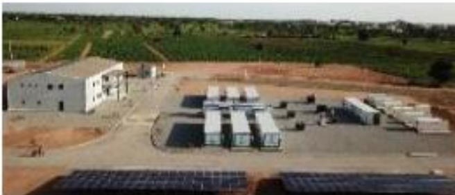
Installation Equipment Area
