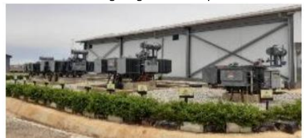
Transformers Installed and Commissioned
