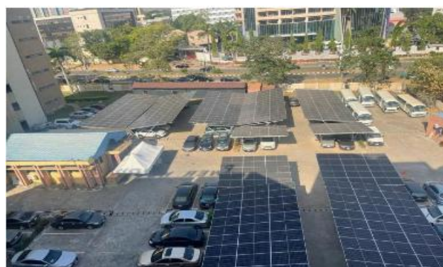
Ongoing Project Abuja and Installed Solar PV Panels at the Junior Staff Car Park
