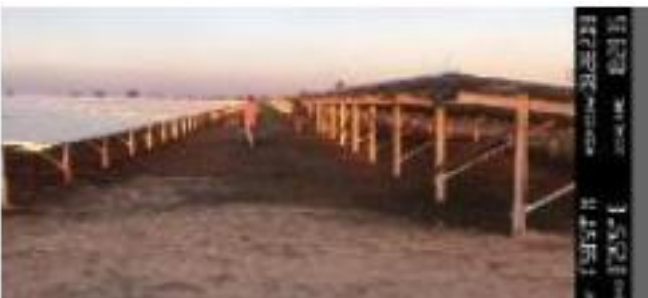
Installed PV Modules
