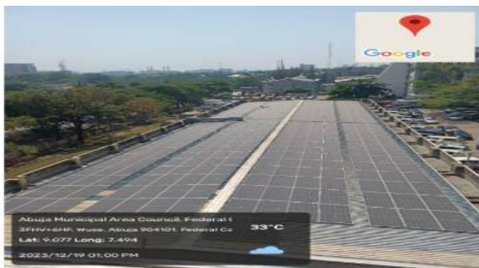
Installed Solar PV modules on the roof of the Extension at Power House, Federal Ministry of Power
