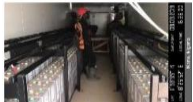
Installed Battery Storage
