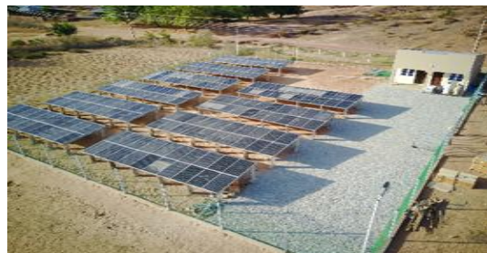
Aerial View of Completed 60kW Power Plant
